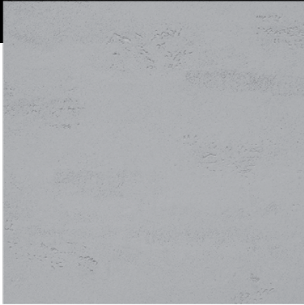
MOA-##-S | Pitted Surface
